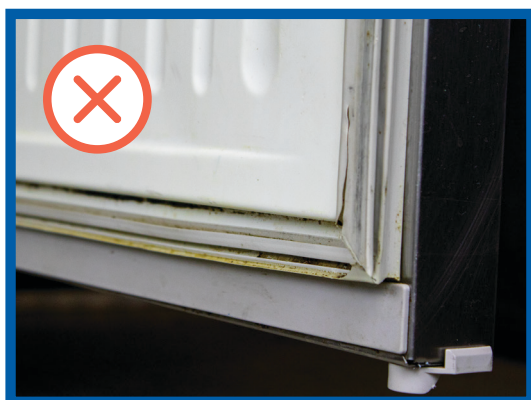
Defect deurrubber koeling
